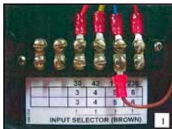
Brown Wire connected to 115VAC
